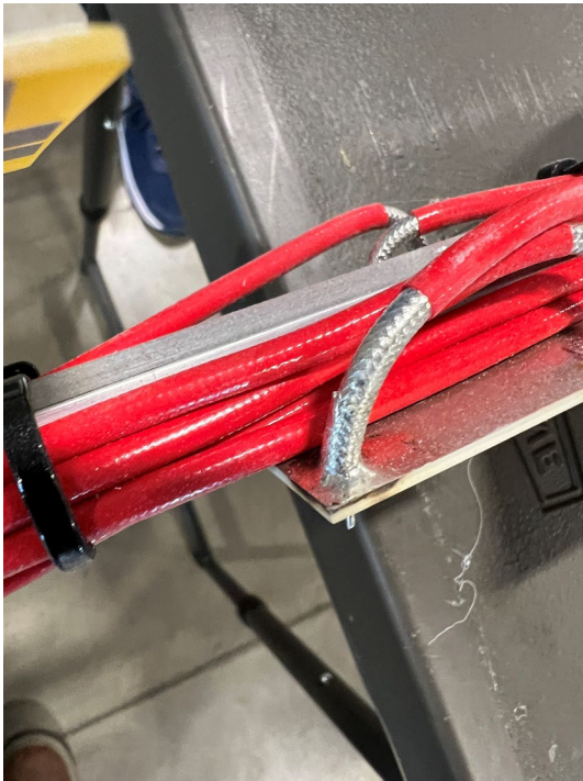
Burned Lifted PCB
